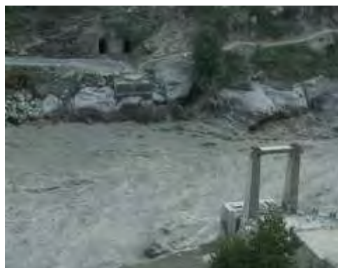
Figure 19: 2005 Floods- Loss of Kharo Bridge
