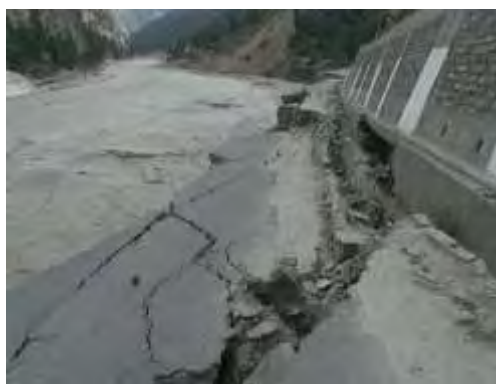
Figure 18: Picture showing damage to roads
