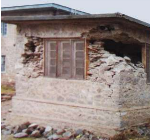
Damage at the corners of the house.
