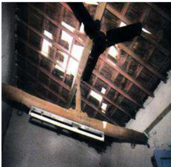
Damage primarily caused by strong winds
