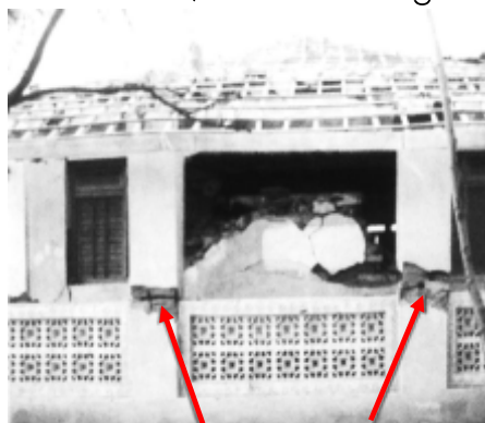
Masonry piers cracking
