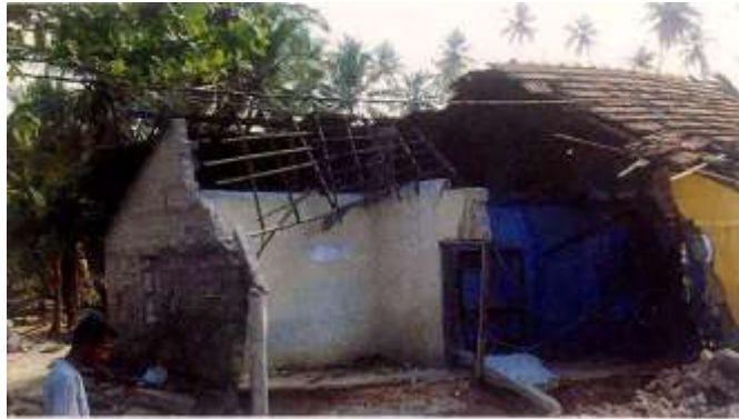
Damage due to strong winds
