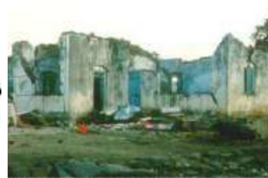
(a) Building with no horizontal lintel band: collapse of roof and walls
