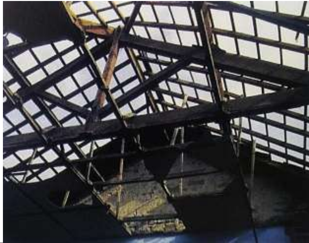
C3 Hazards: Their Severity, Zonation and Impact on buildings NDMA Unnati PIC
