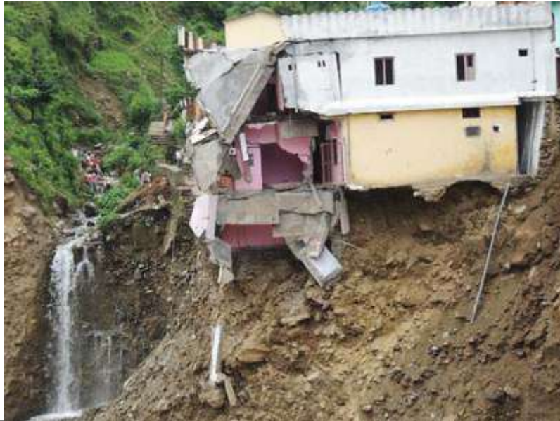
Damage to sub-structure
