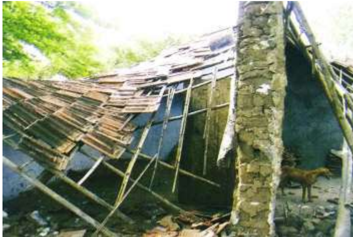
Damage to roof structure
