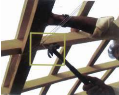
Tie one wire at a time around the joint of strut with rafter or purlin, stretched with a carpenter's hammer.
