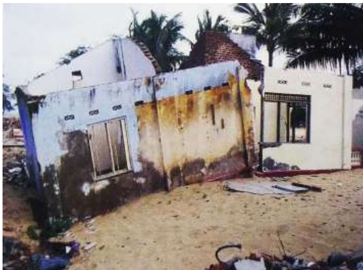
Damage due to foundation settlement
