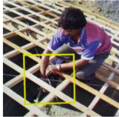
Pre-tension wires by twisting all wires along one diagonal together with a piece of rebar.
