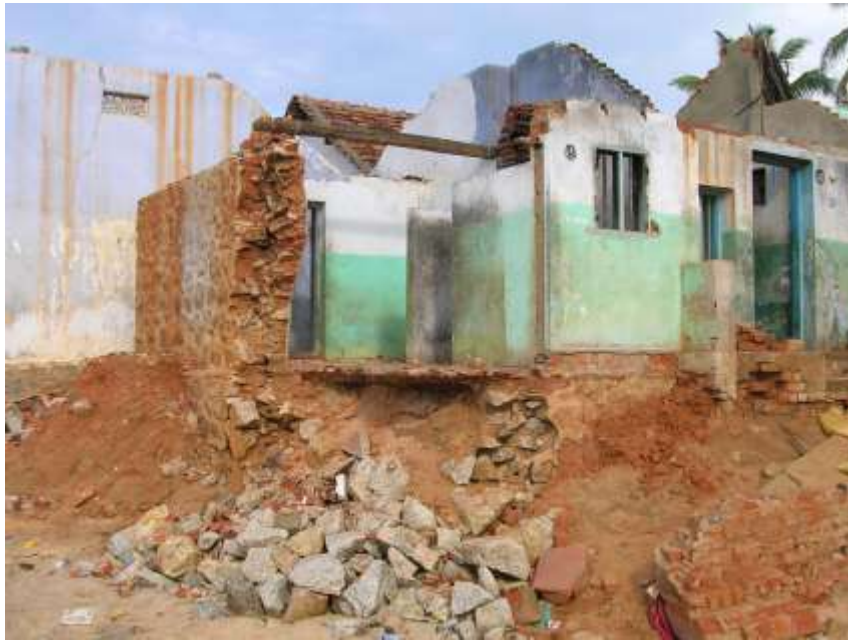
Damage to the substructure and superstructure
