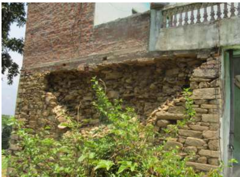
Delamination of stone wall
