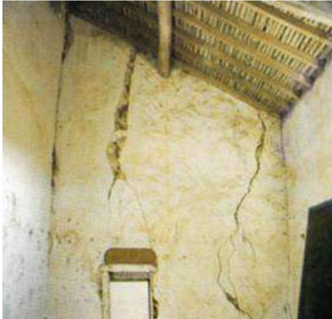
Cracks on the gable wall.
