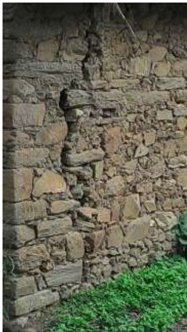
Separation of the wall from stone pier
