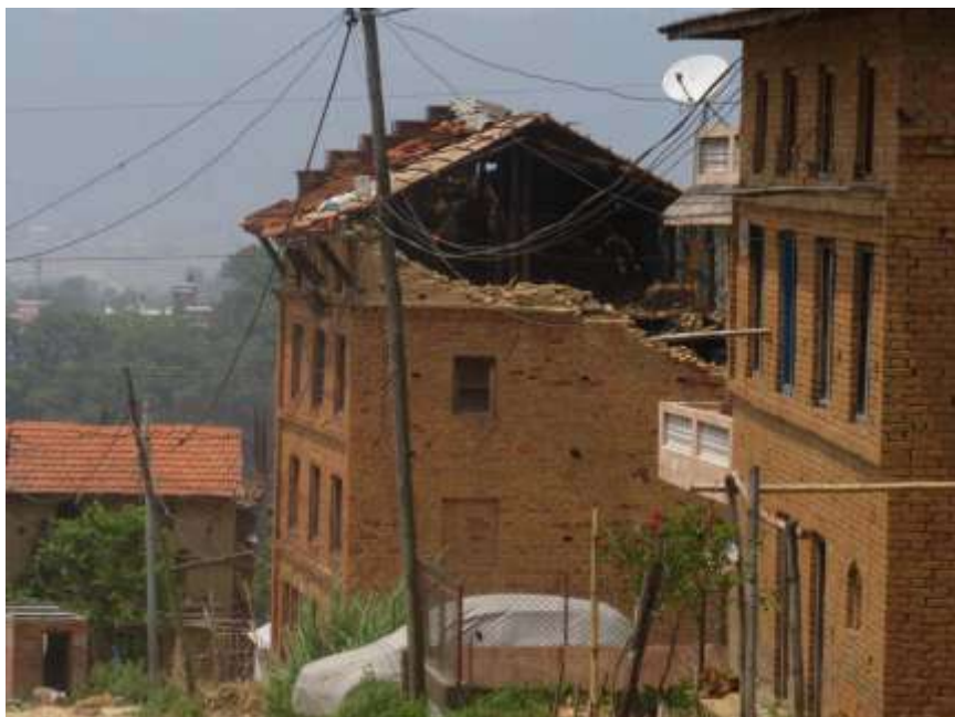
Collapse of the gable wall.
