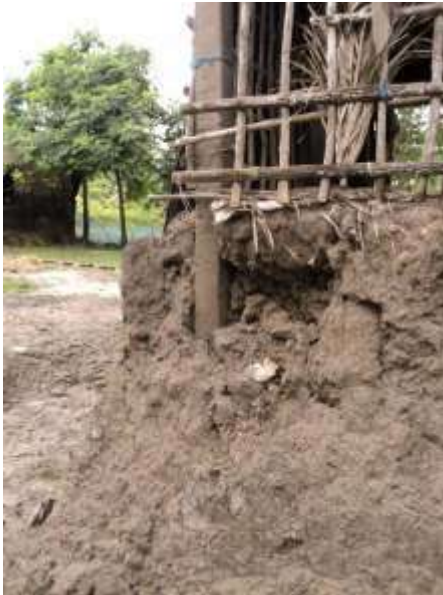
Scouring of foundation
