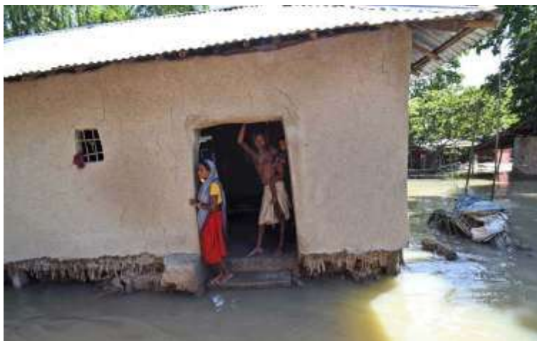
Settlement of foundation.
