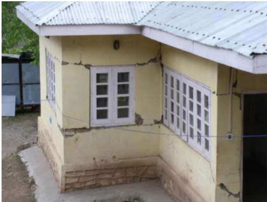
Diagonal cracks around openings
