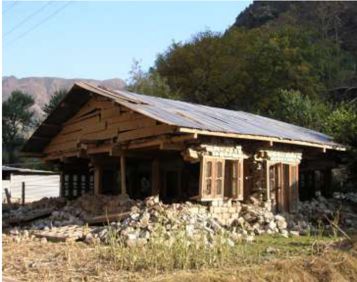
Out-of-plane damage to the exterior wall.
