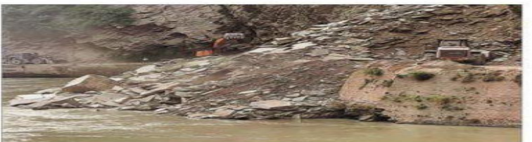
Work underway to clear debris on the Chandigarh-Manali highway near Dwada in Mandi district. PHOTO: JAI KUMAR.
