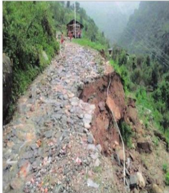
The damaged Neuli-Shanshar road in Sainj valley of Kullu.
