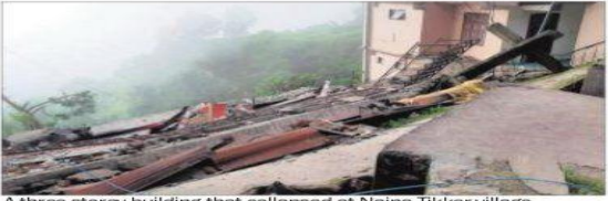
A three-storey building that collapsed at Naina Tikker village.
