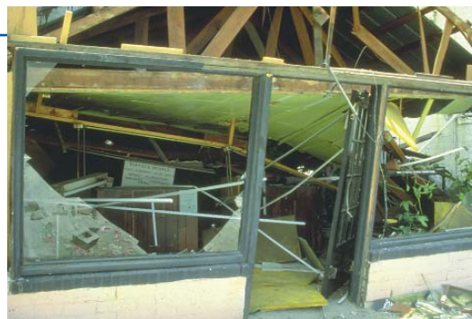
Damaged building, Coalinga, Calif.
