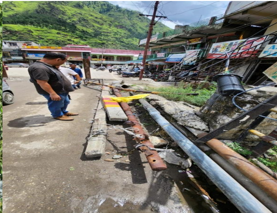
Figure 15. Dismantled poles After the Flood Impact
