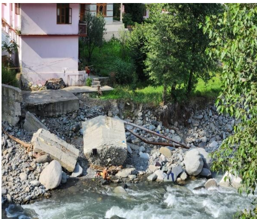
Figure 14 Foundation of The Structure Uprooted
