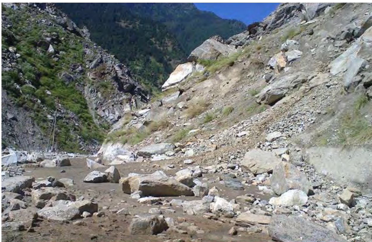
SLIDE BETWEEN KM345-353 ON H-T ROAD
