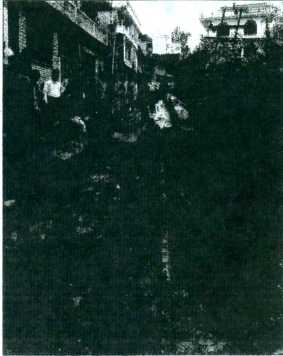
■ The Circuit House road that got damaged during rain in Mandi on Wednesday.
