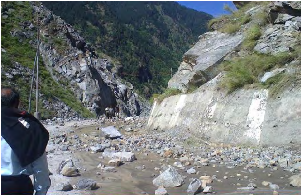
SLIDE BETWEEN KM345-353 ON H-T ROAD
