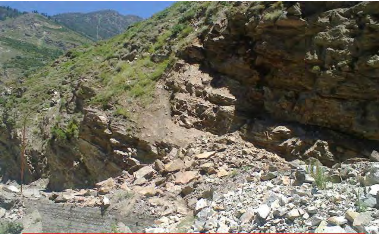
SLIDE BETWEEN KM 336-345 ON H-T ROAD
