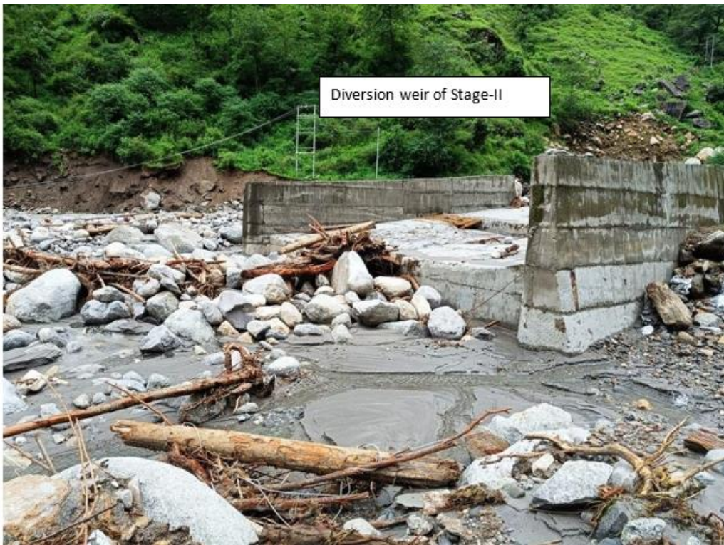
Figure 4 Damaged Diversion weir of Ganvi HEP-II
