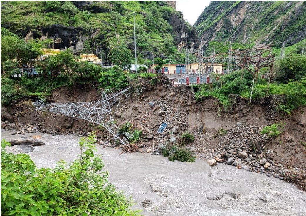
Figure 3. One 66 KV Double Circuit Transmission Tower is damaged near power House of Stage-I
