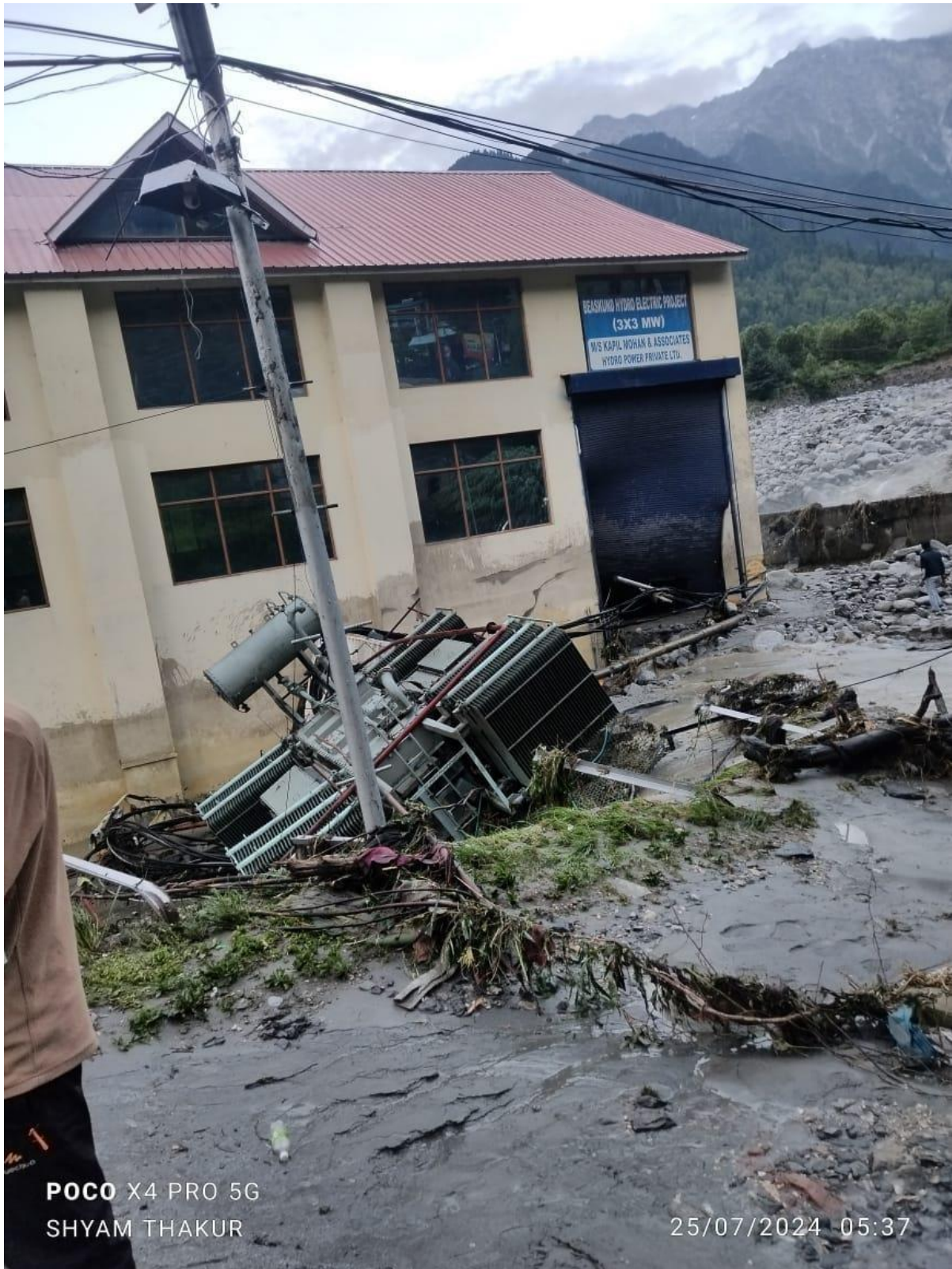
Damage incurred at Kapil Mohan Beas Kund Hydro power project
