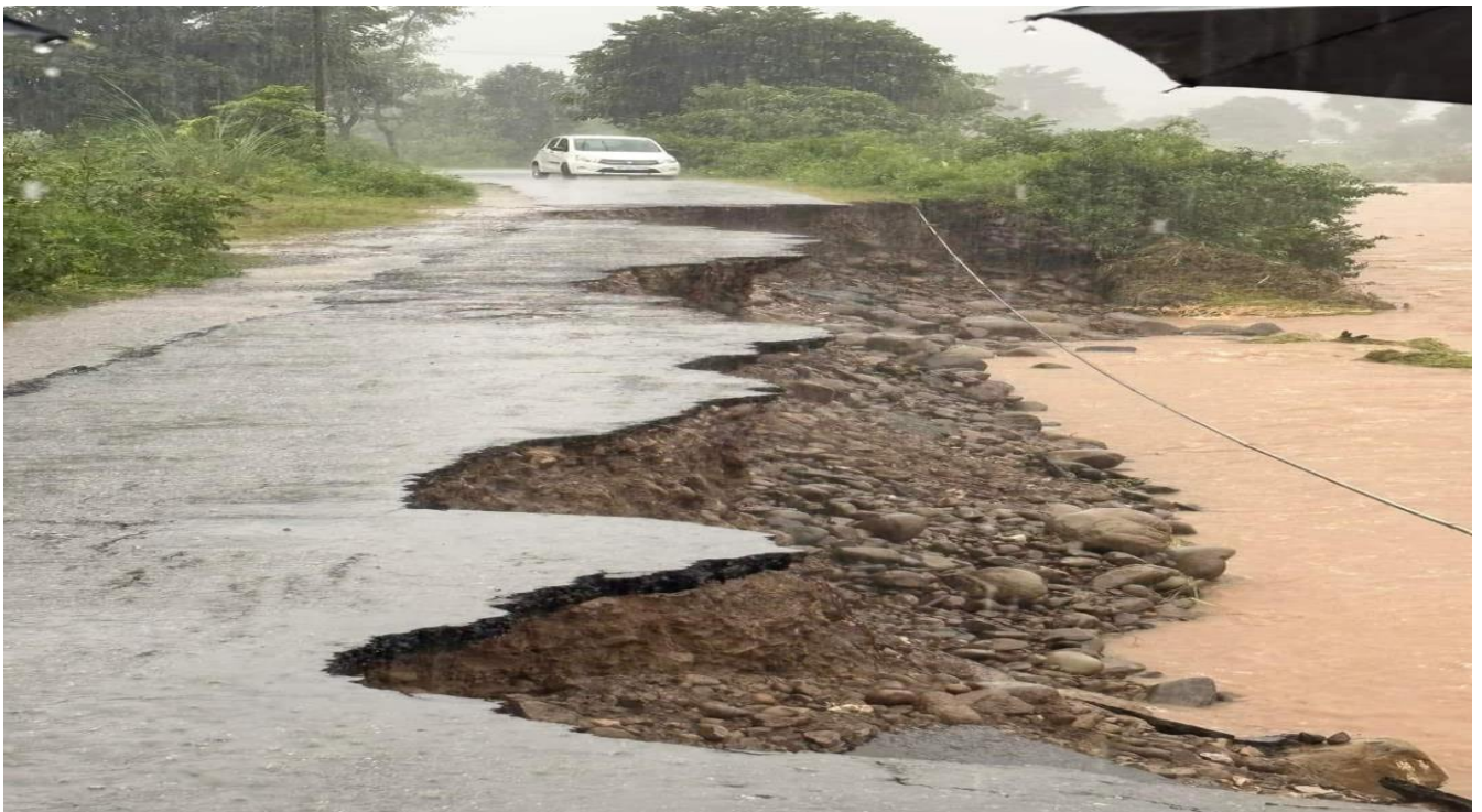
Damages at Sub-Division Paonta Sahib, district Sirmaur
