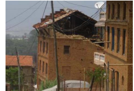
Fig. 2.2.1.2. Impact on gable wall
