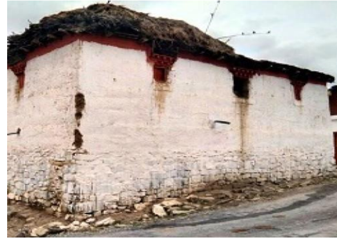
Fig. 6.2.24 Conventional Rammed earth house: Poor EQ safety and required frequent maintenance. Does not have any earthquake bands or corner reinforcement
