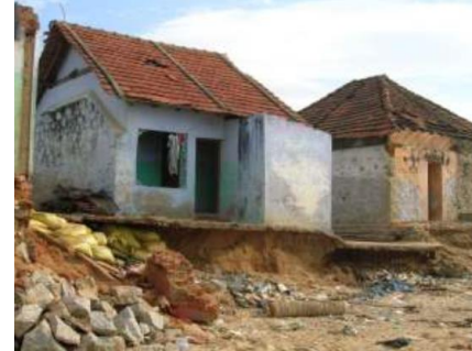
Fig.2.2.3.2. Scouring of foundation
