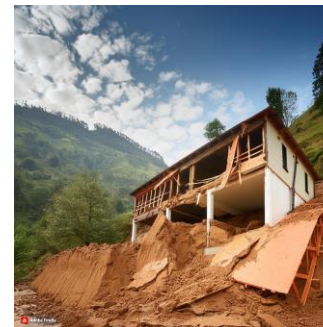
Fig.2.2.3.5. Settlement of foundation
