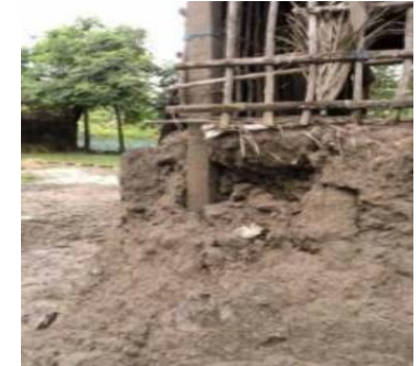
Fig.2.2.3.3 Damage to plinth due to scouring of water
