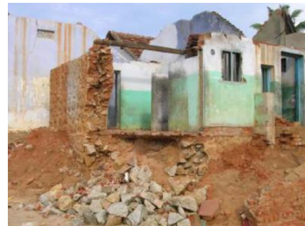
Fig.2.2.3.4. Damage to super structure and the sub structure
