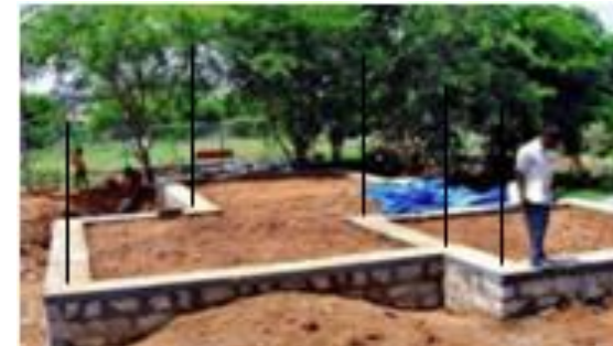
Fig 6.2.21. Continue masonry up to 75mm below the plinth level and then provide RCC plinth band.
