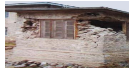
Fig. 2.2.1.4. Impact on corners of the house
