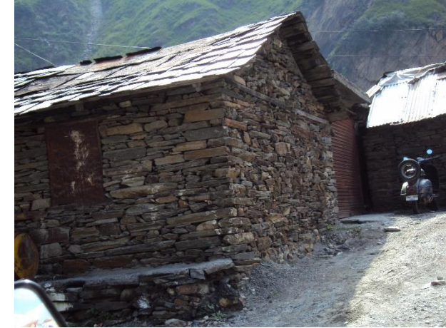
Fig 2.3.2.2. Dry stone masonry is vulnerable to disasters
