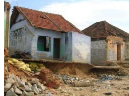
Fig.2.2.3.2. Scouring of foundation
