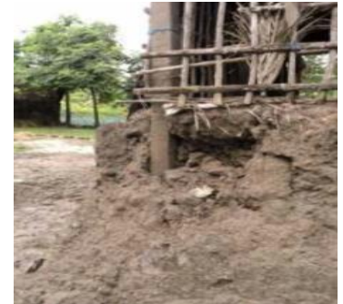
Fig.2.2.3.3 Damage to plinth due to scouring of water
