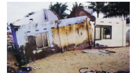
Fig. 2.2.1.5. Impact due to soil liquefaction
