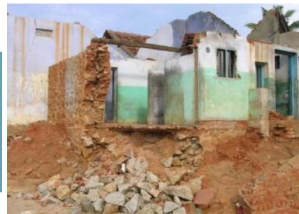
Fig.2.2.3.4. Damage to super structure and the sub structure
