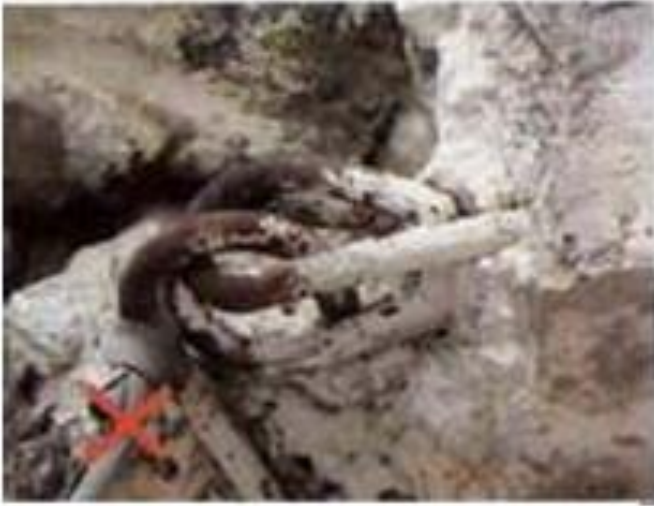
Fig. 7.5.3. Wrong connection of rod through hooks
