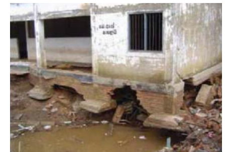
Fig.2.2.3.6. Damage to scouring of soil underneath the plinth
