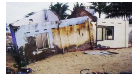
Fig. 2.2.1.5. Impact due to soil liquefaction
