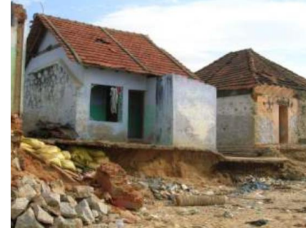
Fig.2.2.3.2. Scouring of foundation
