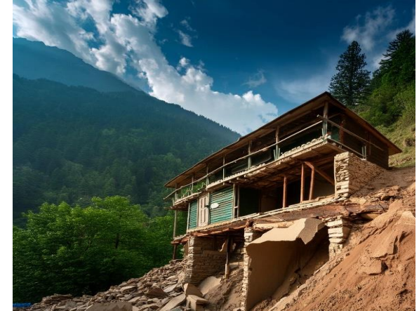
Fig.2.18.Damage to sub structure due to soil erosion
