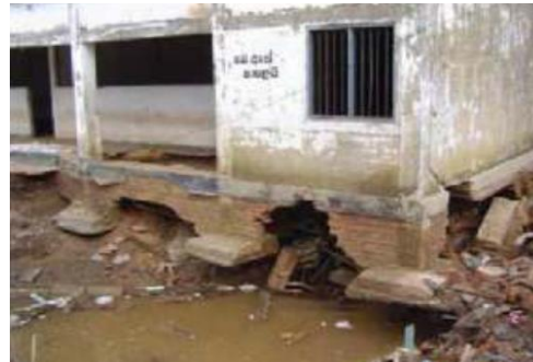
Fig.2.29. Damage to plinth due to scouring of water
