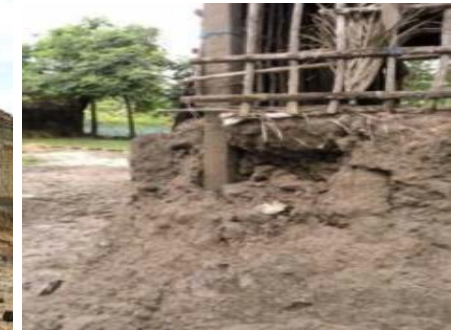
Fig.2.31. Damage to super structure and the sub structure
