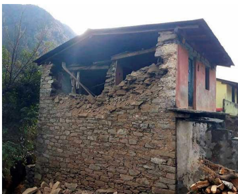
Fig. 2.15. Out of plane damage to wall
