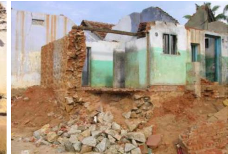
Fig.2.28. Damage to scouring of soil underneath the plinth
