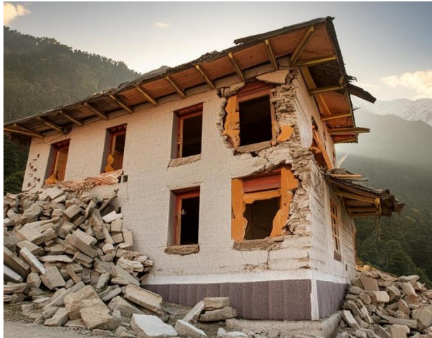
Fig.2.13. Cracks at openings that are too close to corners
