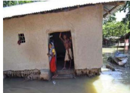
Fig.2.26. Scouring of foundation
