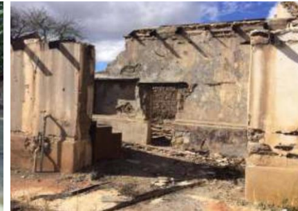
Fig.2.27. Settlement of foundation
