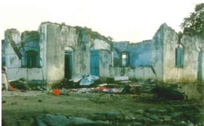
a) Collapse of a Building with no vertical and horizontal lintel bands
