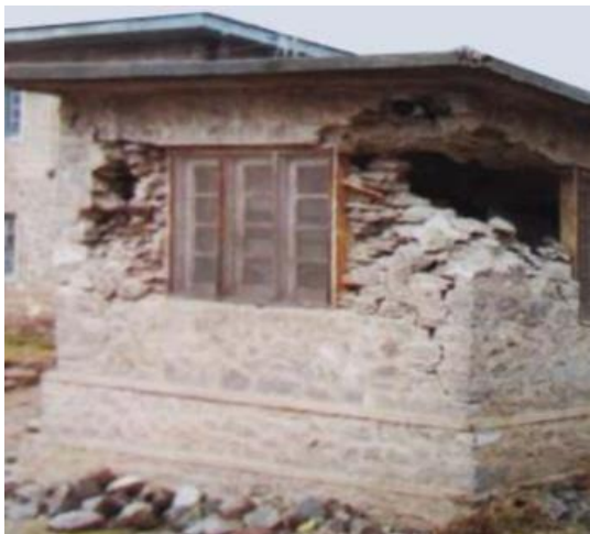
Fig. 2.12. Collapse of masonry
