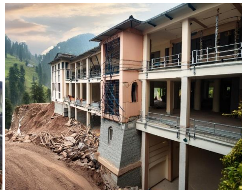
Fig.2.16. Damage due to foundation settlement
