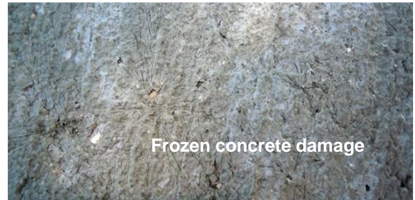
Fig.6.8. Frozen concrete damage
