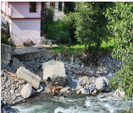
Figure 14 Foundation of The Structure Uprooted
