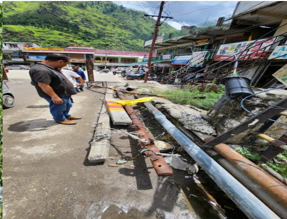
Figure 15. Dismantled poles After the Flood Impact
