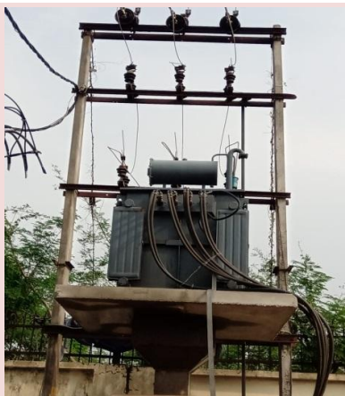
Figure 13 Plinth mounted prefabricated
