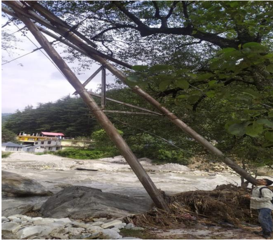
Figure 12 Deformed Poles Due to Flood
