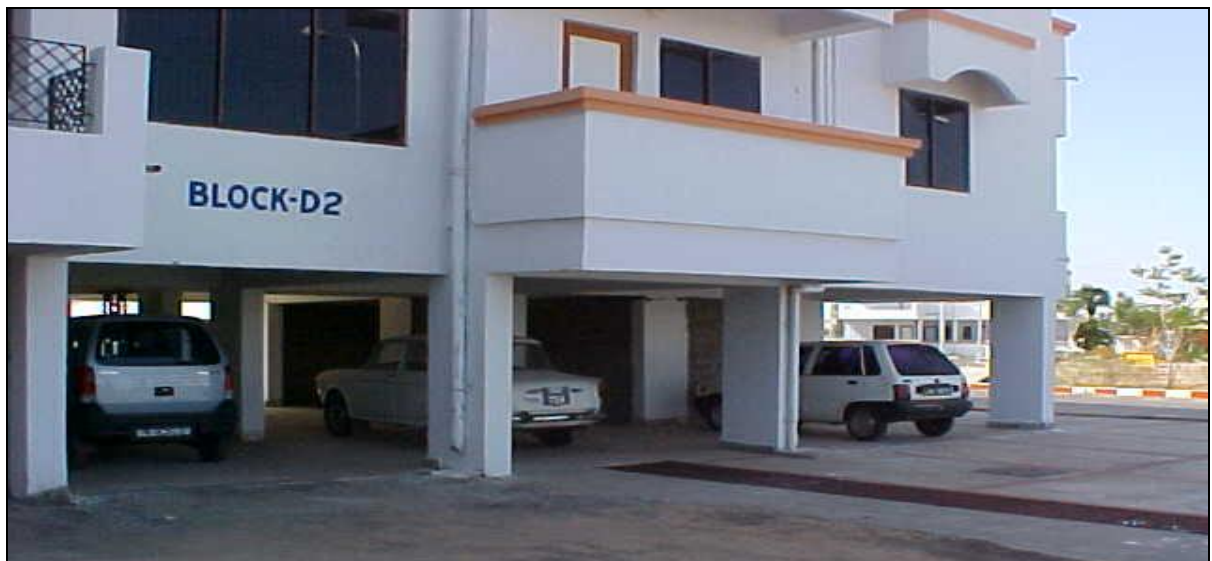
Figure 5: RC Frame Buildings with columns in open ground storey of 230mm width
