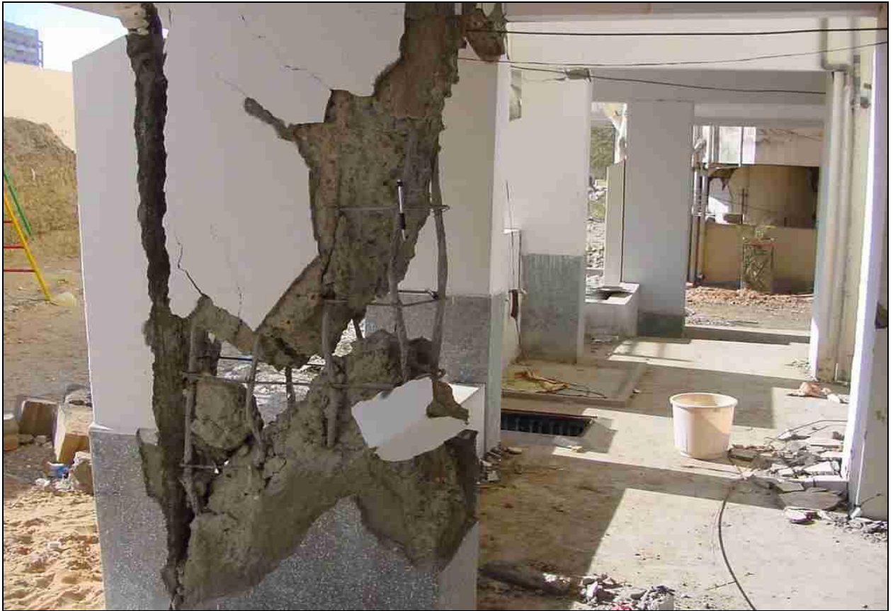
Figure 6: 230 mm wide columns in ground storey of RC Frame Buildings: damaged column in Bhuj town during 2001 Bhuj earthquake
