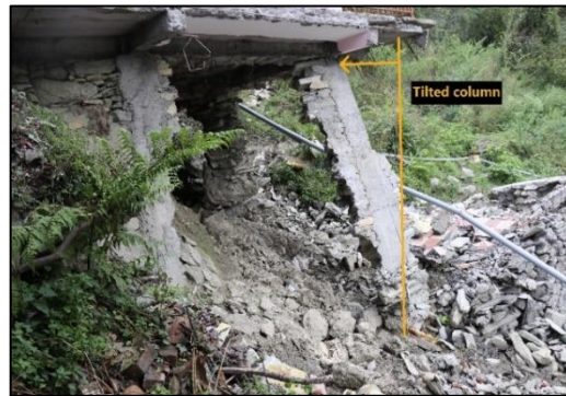
Fig. 38. Tilted column of school building.
