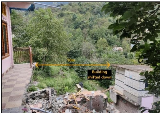
Fig. 37. Building shifted down due to subsidence.
