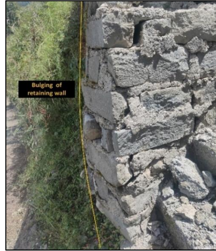
Fig. 31. Bulging of retaining wall.
