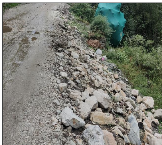
Fig. 27. Damaged Road filled with local material.
