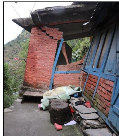
Fig. 15. Tilted house with large cracks.
