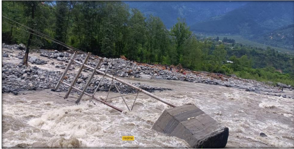
Fig. 62. Damaged Bridge located at Jagatsukh
