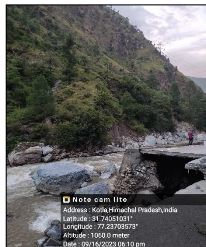
Fig. 50. Loss of pavement material due to erosion.
