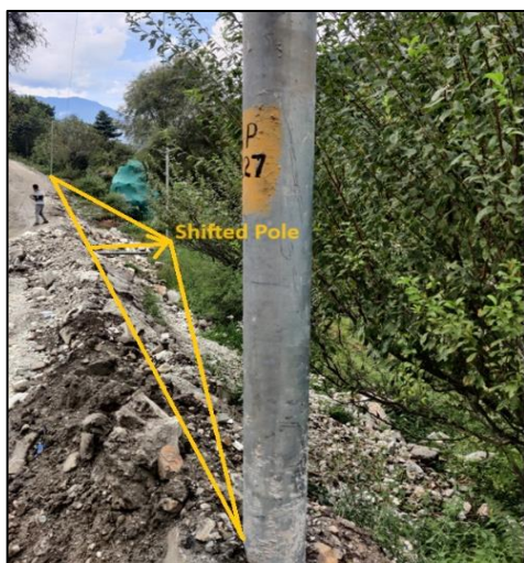
Fig. 26. Shifted pole due to subsidence.
