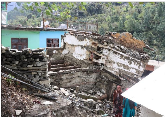
Fig. 24. Damaged house made of wood and stone.
