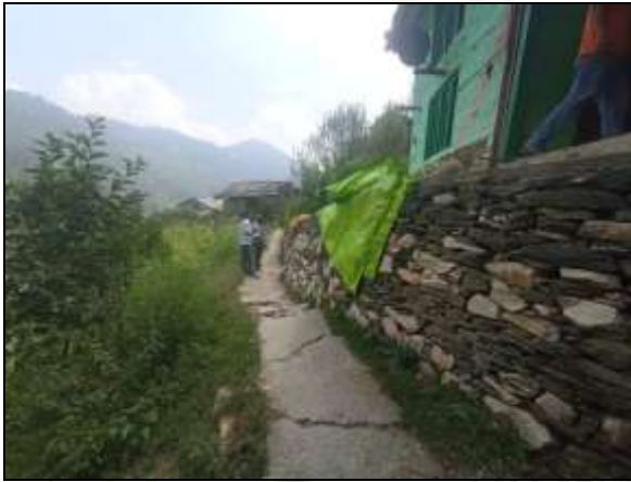
Fig.48; Ground cracks and partially damaged retaining wall.
