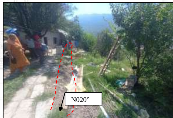
Fig.14; Ground cracks observed at Banontar Kharahal
