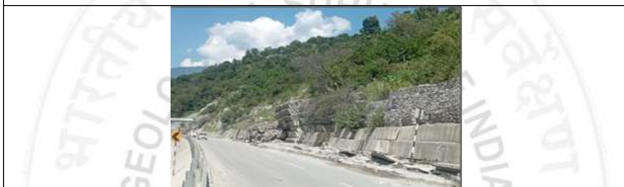
Fig.3 Damage retaining structures along NH-3.
