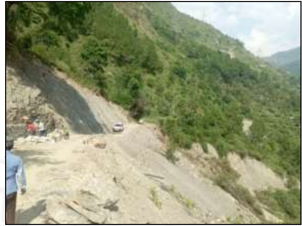
Fig.38; Road subsidence along Machine Nala landslide.
