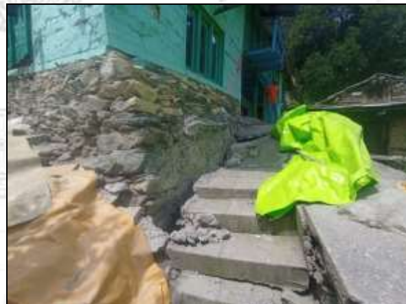
Fig.51; partially damaged houses Mourod
