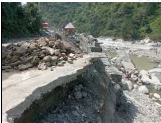
Fig.40; Severe road damaged near Thana Sainj.
