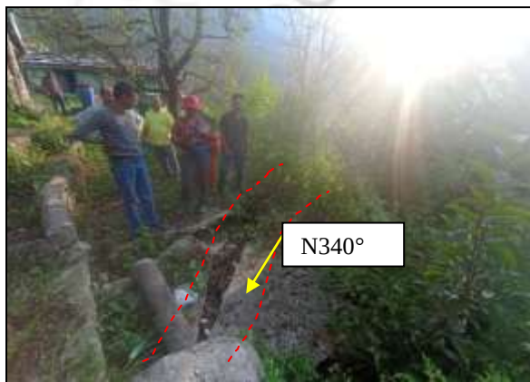
Fig.19; Ground cracks at Garsa village.
