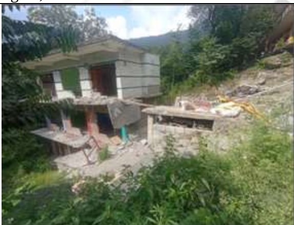
Fig.2. Damaged Sarswati Vidya Mandir Sr.Sec. School
