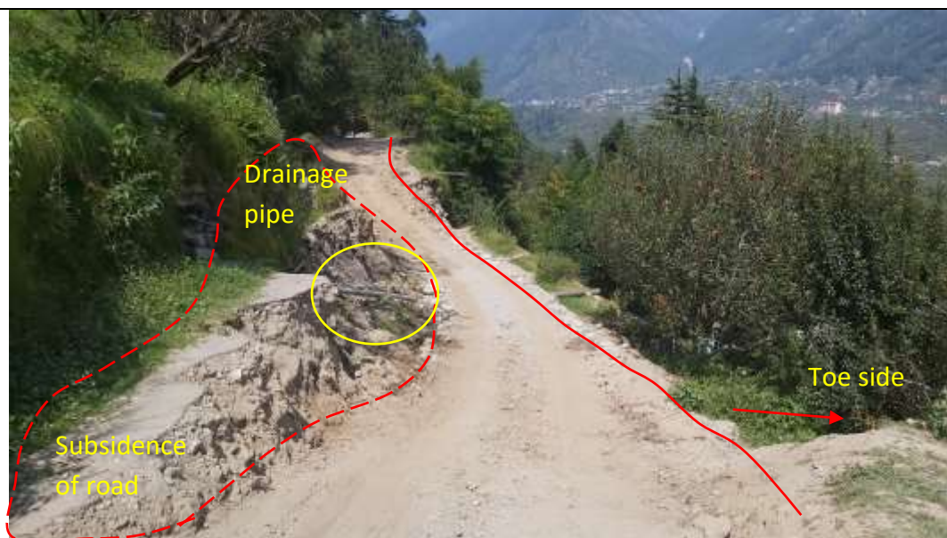
Fig.1. Subsidence of road observed in Shaleen village
