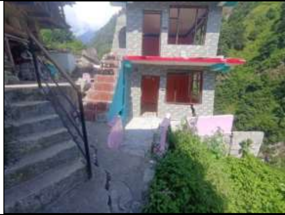
Fig.2. Crack on civil structures
