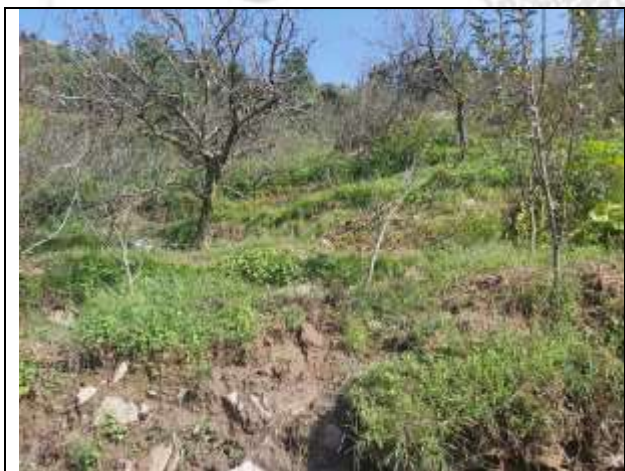
Fig. 70. Debris slide observed in Chehva village on the road side of NH 305
