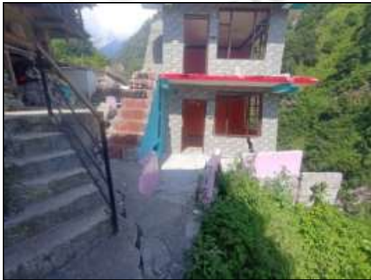
Fig.23; Crack on civil structures at Barauna village
