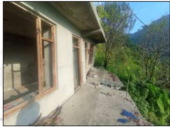
Fig.18; Damaged house at Garsa village.
