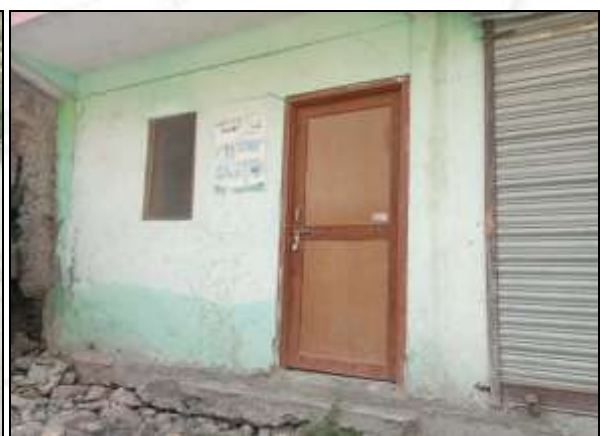
Fig.59; Cracks on walls at Kartah.
