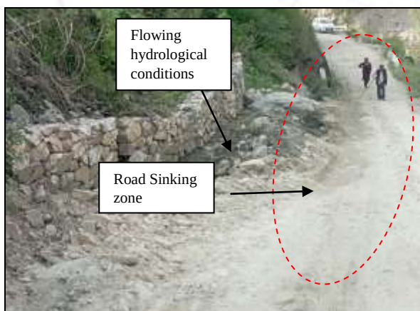
Fig.58; Road subsidence at Kartah
