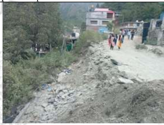
Fig.3. Damaged road stretch
