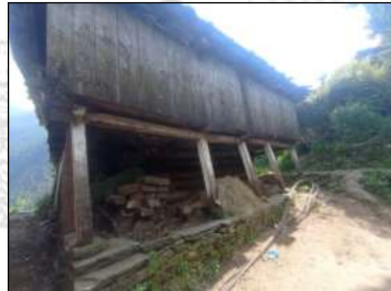
Fig.24; Tilting of houses at Barauna village.
